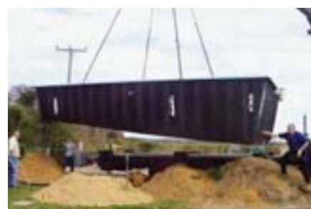
The pool is lowered by crane into place: the finished perfect pool. © Multiforma
